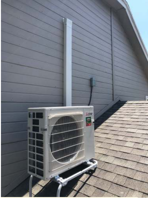
New Mitsubishi Outdoor Unit
