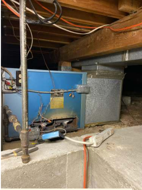
Old Furnace In Crawlspace
