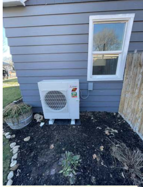
New Mitsubishi Heat Pump
